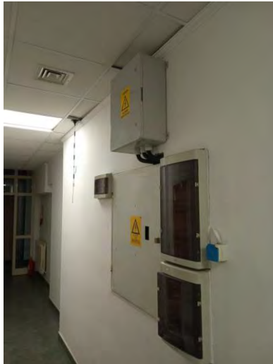
LV Power units
