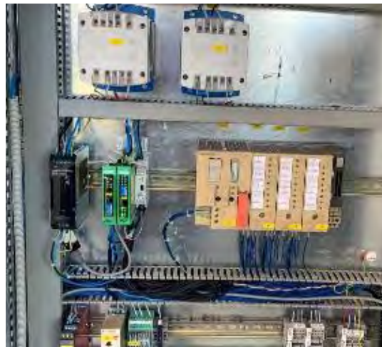
Figure 6-35 Setup of Modbus devices at Rio facility site
