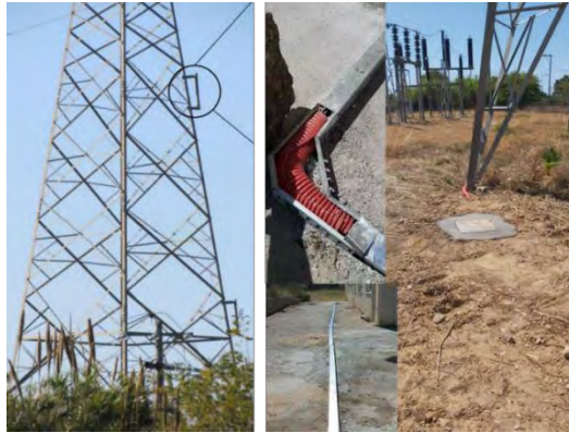
Figure 6-7 Deployments at the ADMIE facility (see point B1 in map above)
