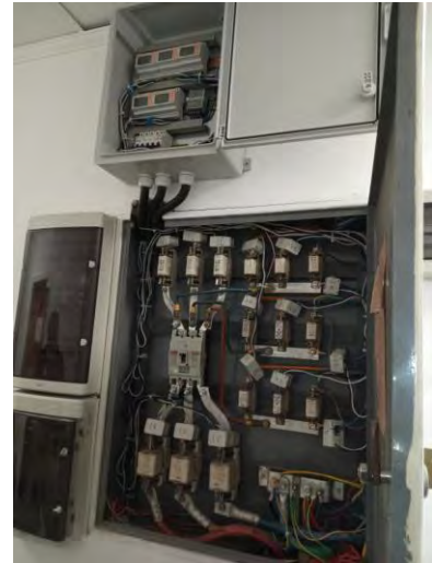
LV in buildings
