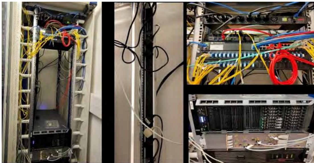
Figure 4-4 MShed Server room equipment
