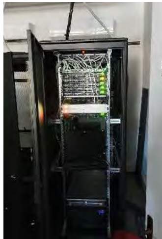
Figure 6-8 Part of the UoP data centre (see point A in the maps above)
