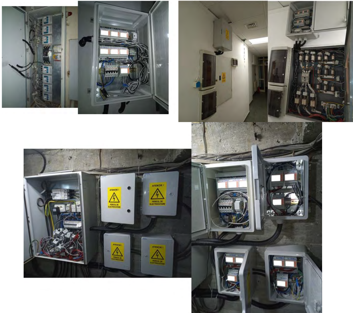
Figure 5-5 Measurement devices installed on 3 sites from Alba Iulia
